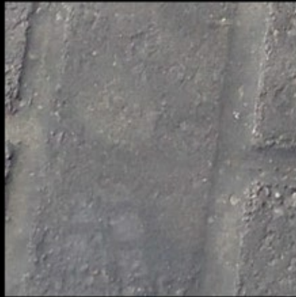
Polished paving blocks at Juffair traffic light.
